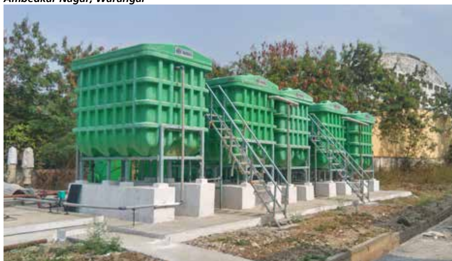
Image 1: Moving bed biofilm reactor technology based sewage treatment plant at Ambedkar Nagar, Warangal
