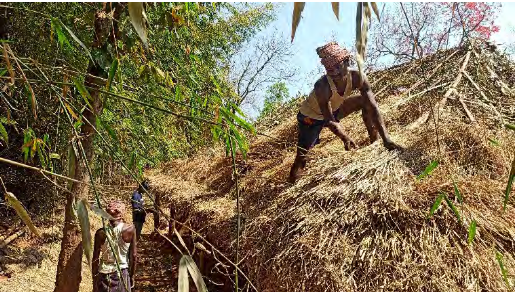
The thatch bundles are orderly placed over the layer below, to avoid gaps in the roof
