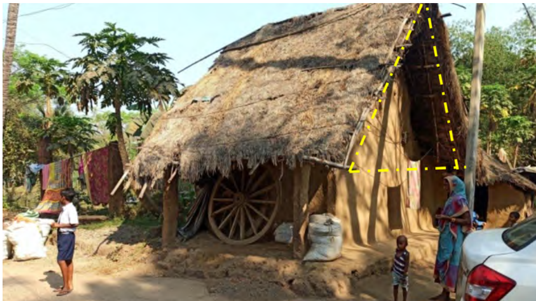
Building with increased slope of roof, which is a common feature in most of the vernacular housing in the coastal region
