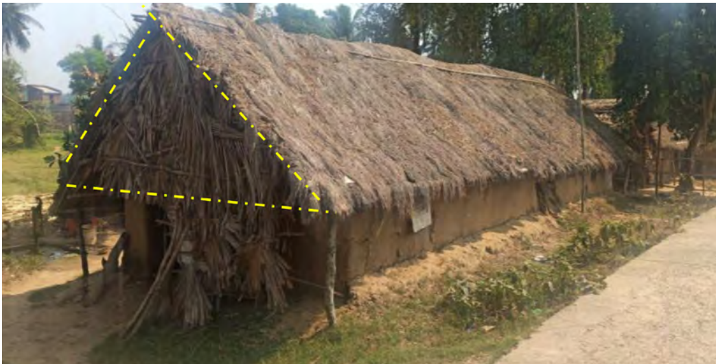
Pitched roof with increased slope and longer side of the building aligned with wind
