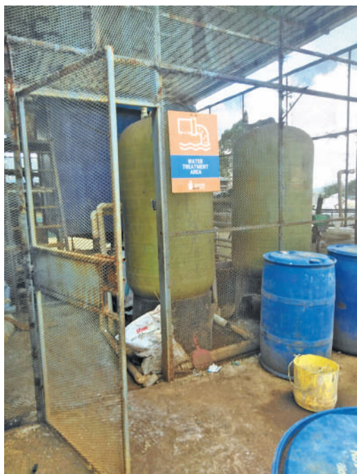
Water treatment plant within the the takataka solutions facility
