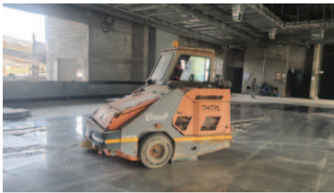
Mechanical sweeping machine at NCRTC stations
