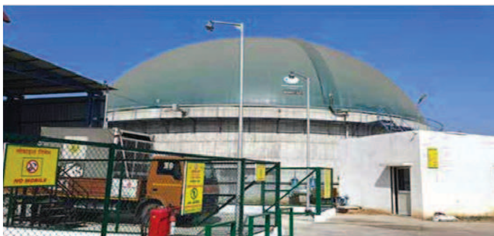
Biogas digester with a total capacity of four tonnes per day (TPD)
