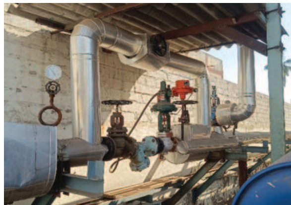
Common boiler pressure decreasing system inside the industry
