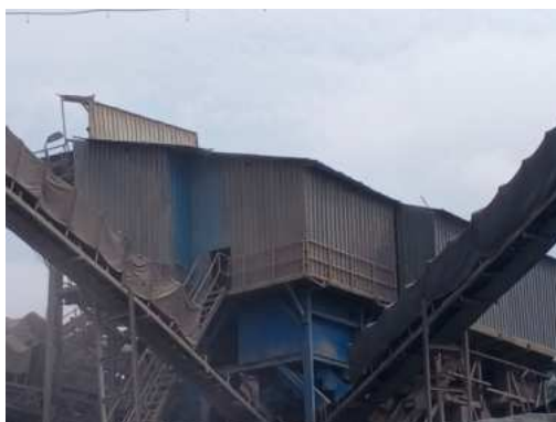
Covered screen with door arrangements
