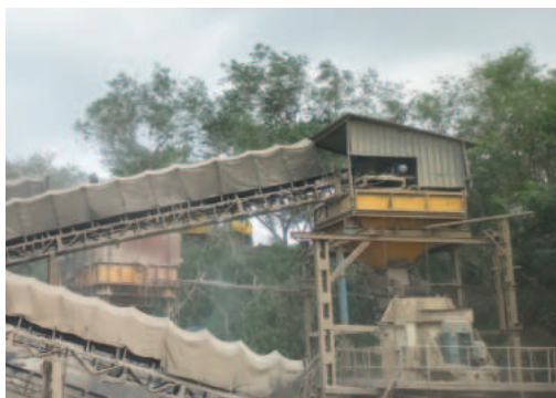
Covered conveyor belts
