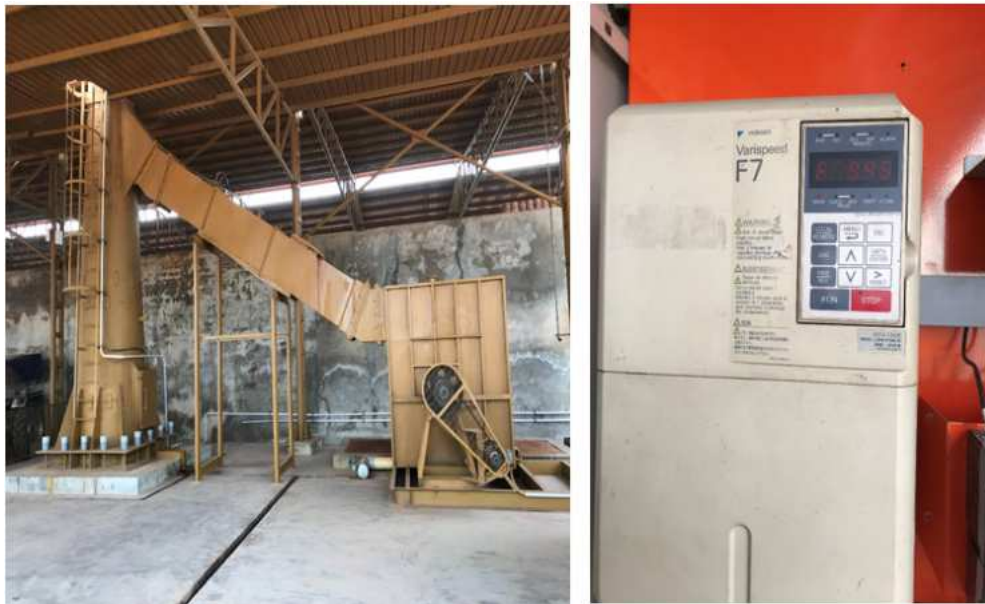
Mild steel stack with a variable frequency drive (VFD) fan instrumental panel
