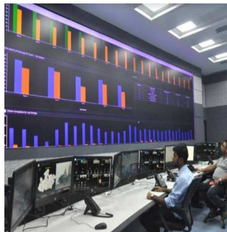
Integrated command and control centre
