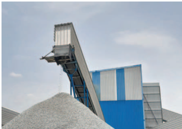
Covered conveyer belt
