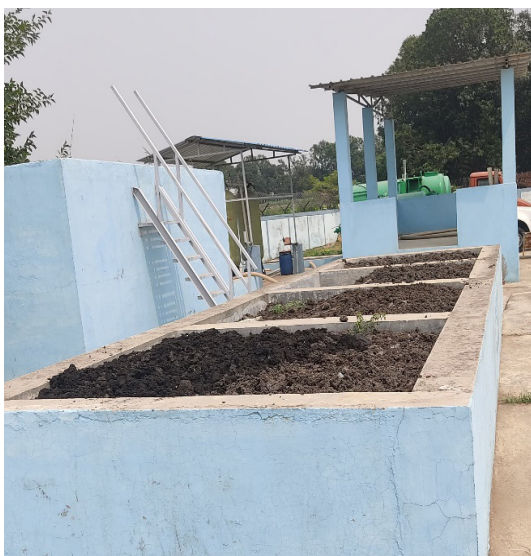
Sludge drying beds full of biosolids (overflow) in Badaun city
