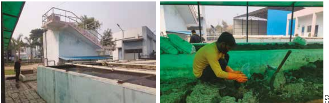
The filtrate tank and sludge drying bed in Prayagraj
