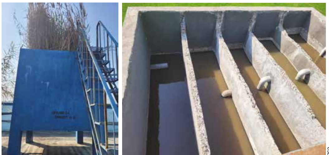
Primary (baffled reactor) and secondary (wetland) treatment modules in Khurja FSTP
