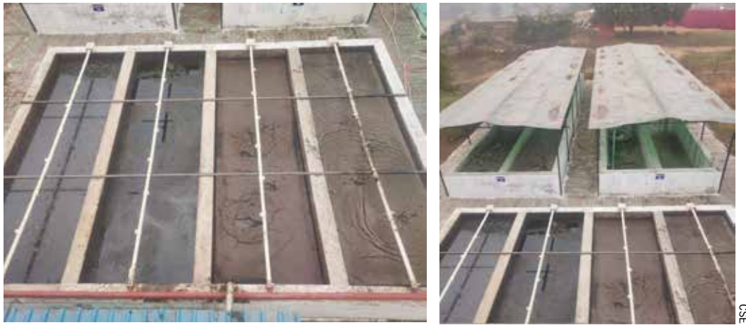
The primary treatment and drying beds in Varanasi
