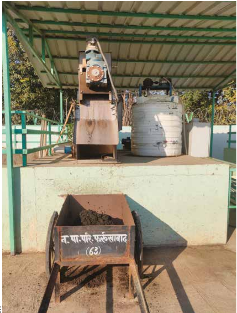
The primary treatment stage in Farrukhabad
