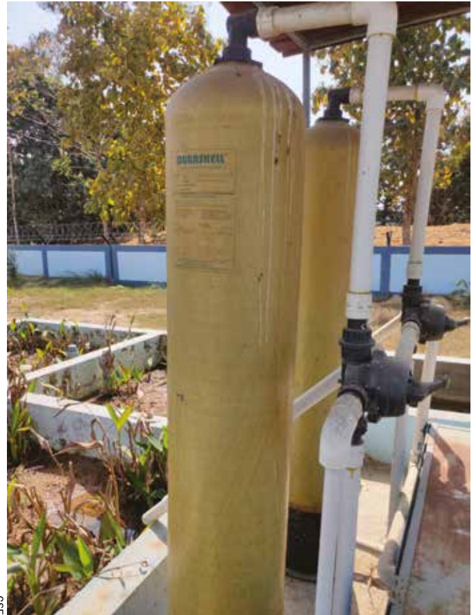
Filtration module in the Bahraich FSTP
