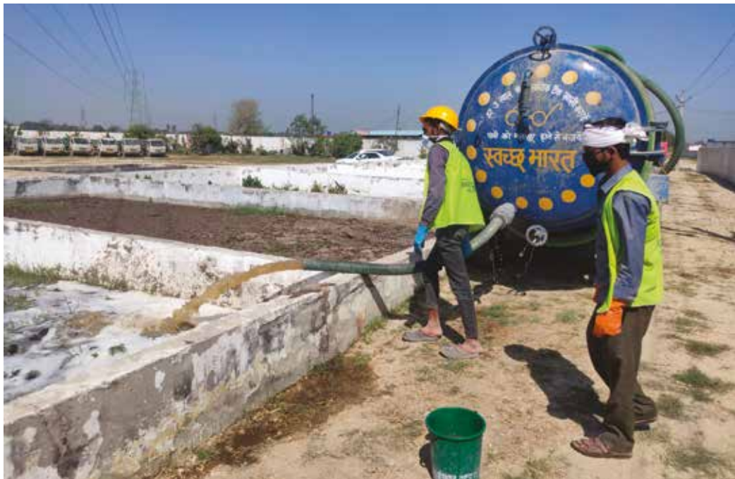
Decanting the faecal sludge in unplanted drying bed
