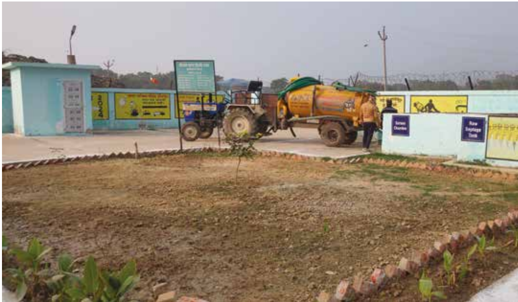
Desludging the faecal sludge in the screening chamber initiating the preliminary stage
