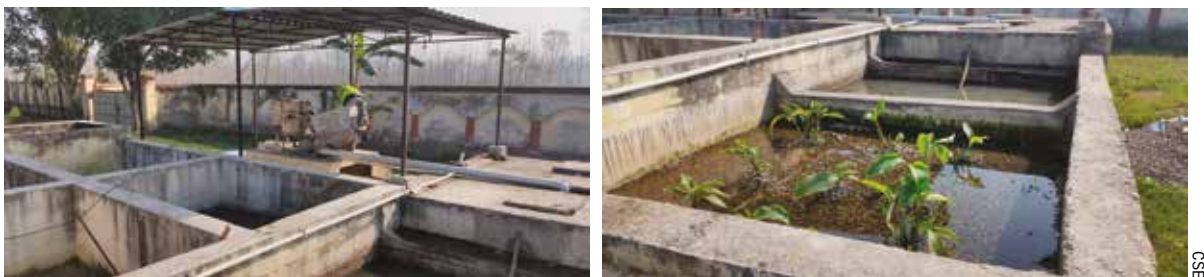
The primary treatment along with the tertiary treatment modules in Rampur
