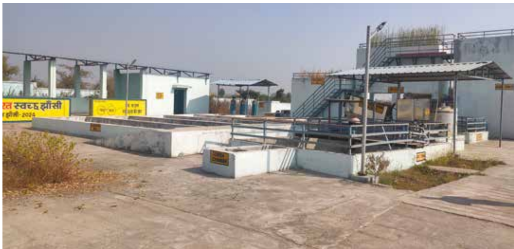
Different treatment modules in Jhansi 32 KLD FSTP
