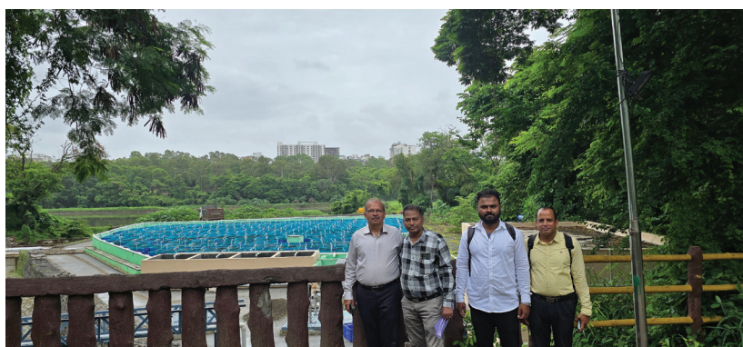
A Tiger Biofilter-Based Technology treatment plant has been installed to treat sewage before releasing into Katraj Lake
