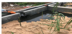
Raw Faecal Sludge
