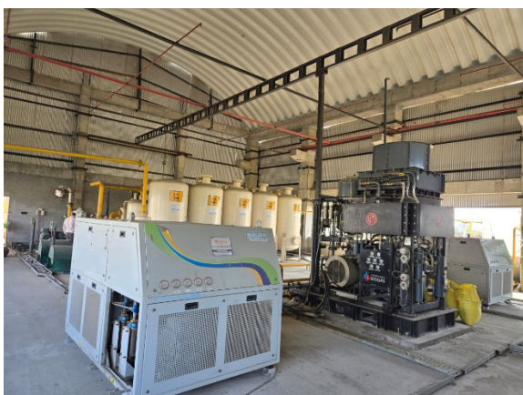
The compression unit at the plant
