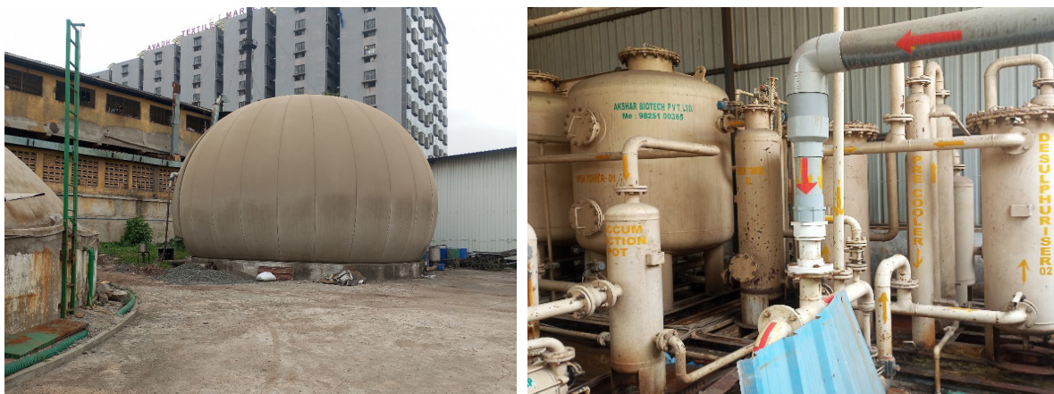
CBG storage area (on left) and the filtration area
