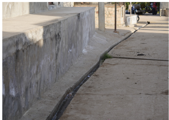
Drain of irregular shape and size in Nawgura village, Rani block
