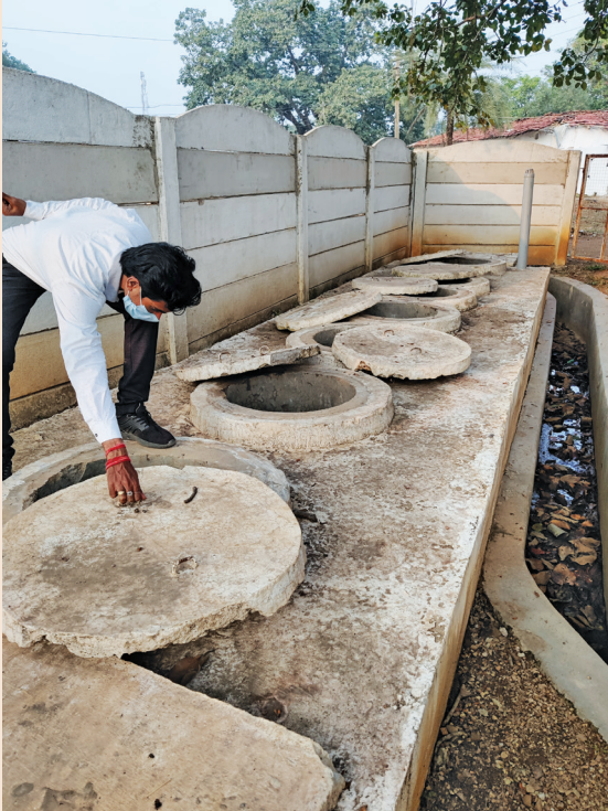
Greywater treatment plant in Ghughwa village
