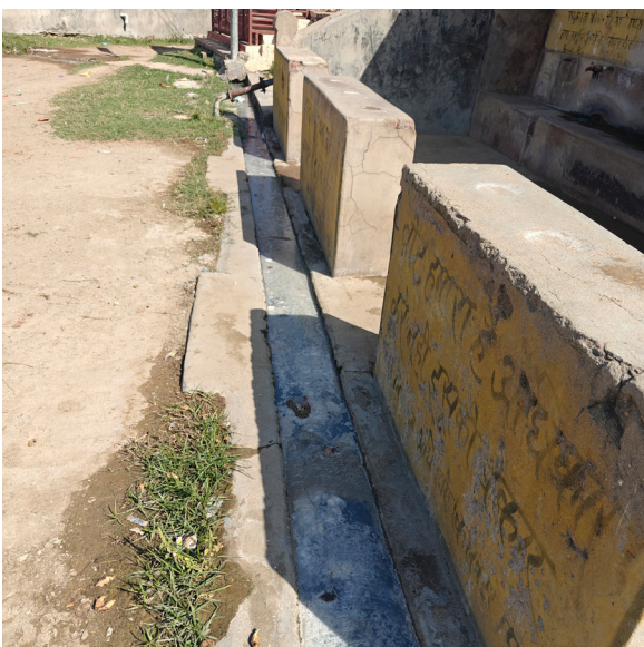
Drain of inadequate depth in Basant village, Sumerpur block
