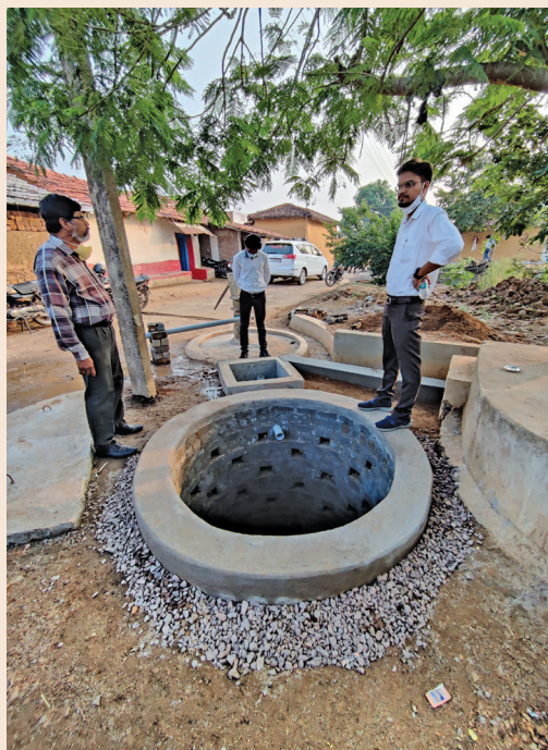
Community-level modified leach pit with nahani trap and silt chamber in Patora village
