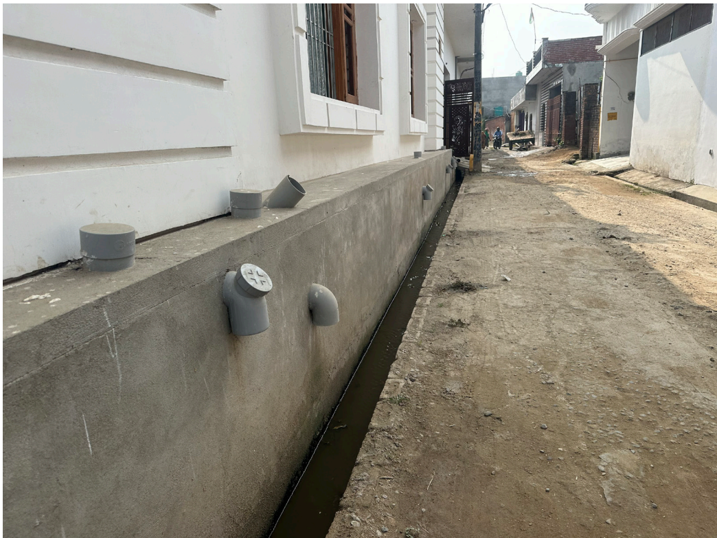
Household wastewater outlets in Ward 7
