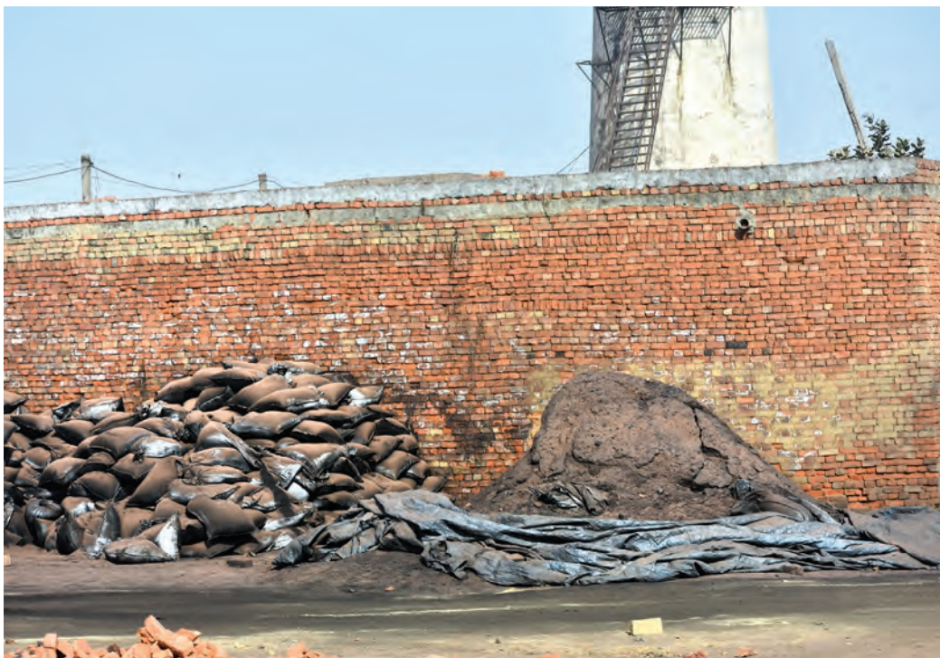
Unplastered outer wall of a brick kiln with adjacent fuel storage area
