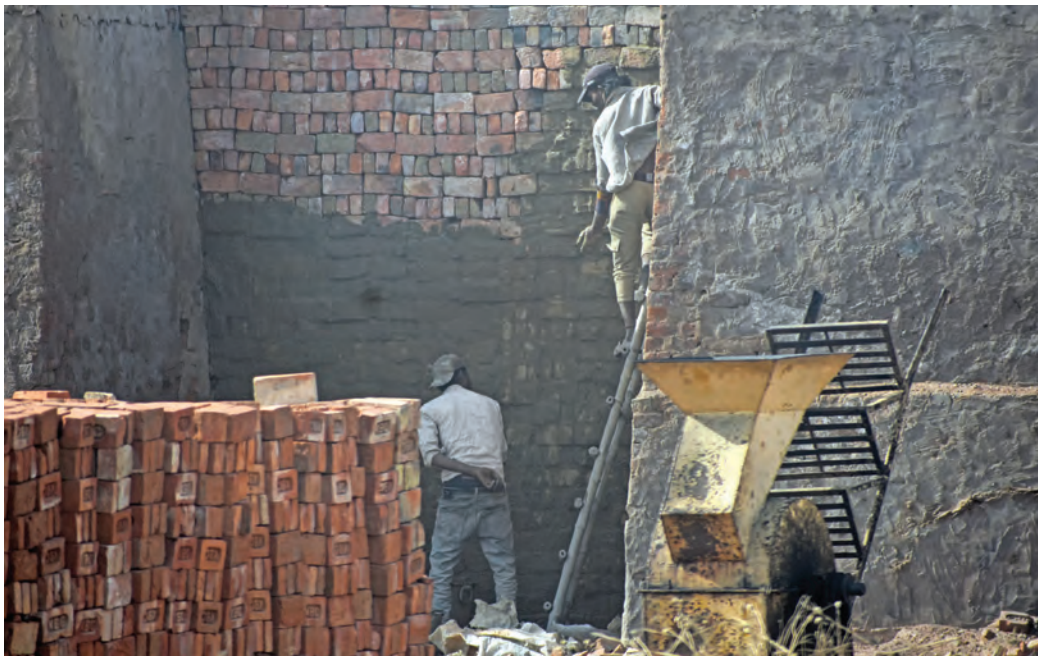
Mud plastering being carried out on the outer wall of a brick kiln
