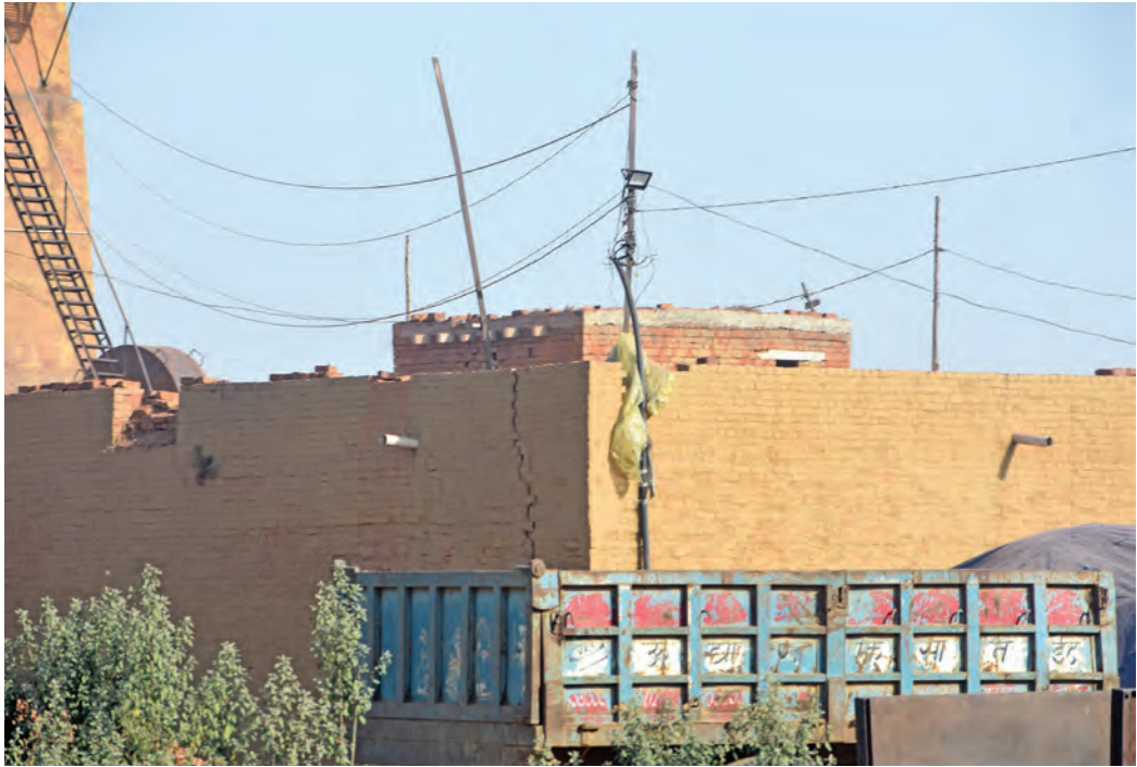
Cracks observed on the outer wall of the brick kiln
