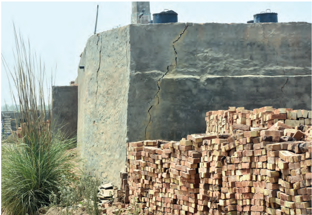
Structural cracks on the exterior wall of the brick kiln
