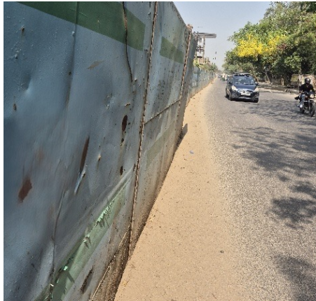
Dust at the base of wind breakers to be cleaned
