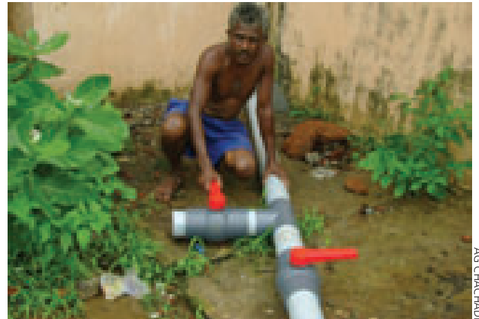
First flush device in use in the roof top RWH site on campus
