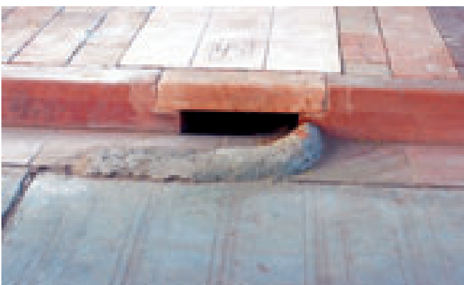
Inlet for road side drainage
