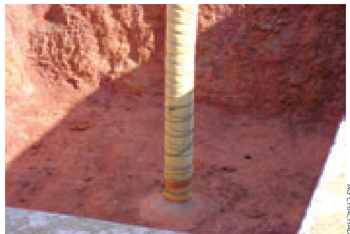
Deep recharge bore well
