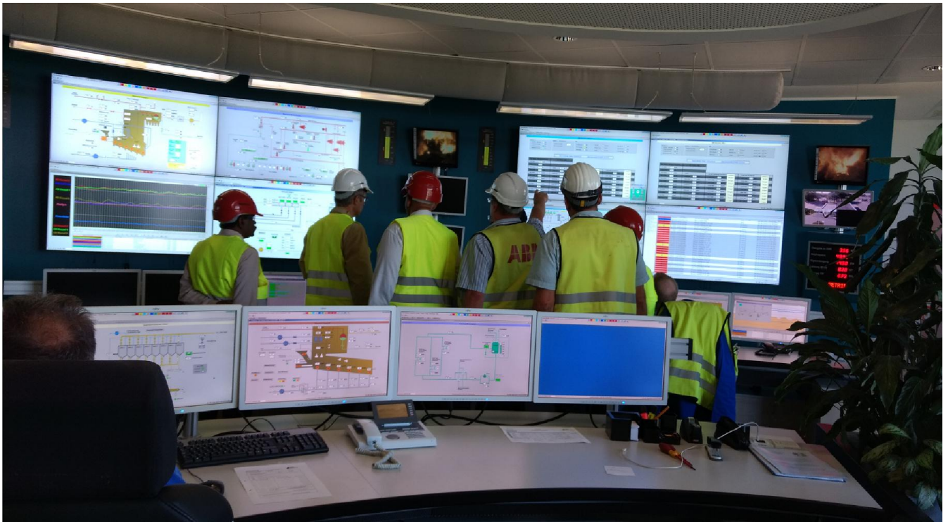
Team checking CEMS data in plant's operation control room at EGK, Krefeld
