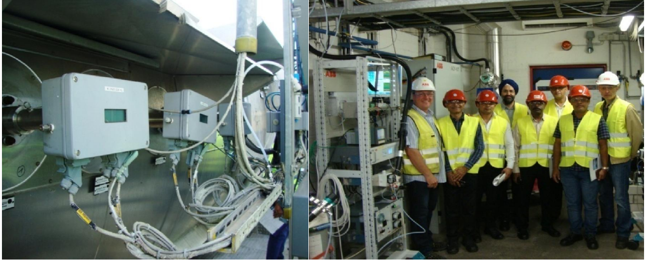
Probes installed in duct before flue gas treatment (left); the team visiting CEMS house (right) at EGK, Krefeld
