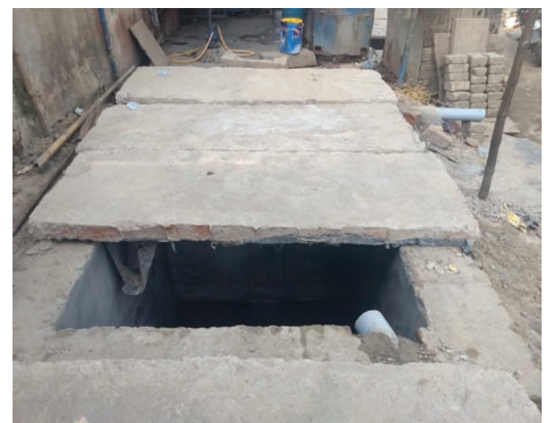
Figure 1: Septic tank having outlet connected to open drain
