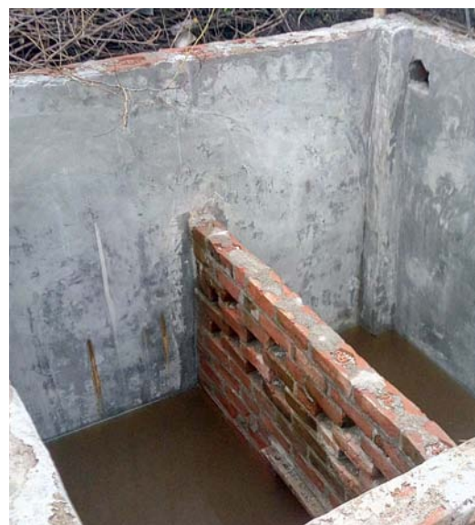
Figure 1: Septic tank connected to open drain
