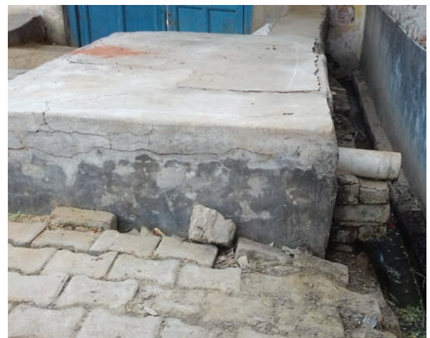
Figure 1: Septic tank of a household connected to open drain
