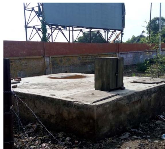
Figure 1: Septic tank connected to open drain
