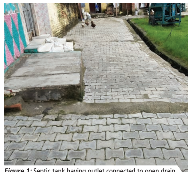
Figure 1: Septic tank having outlet connected to open drain
