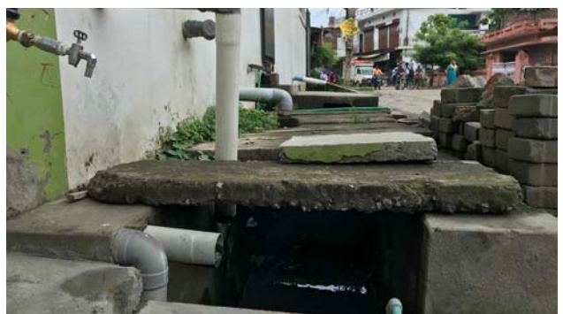
Figure 5: SN from septic tank discharging into open drain
