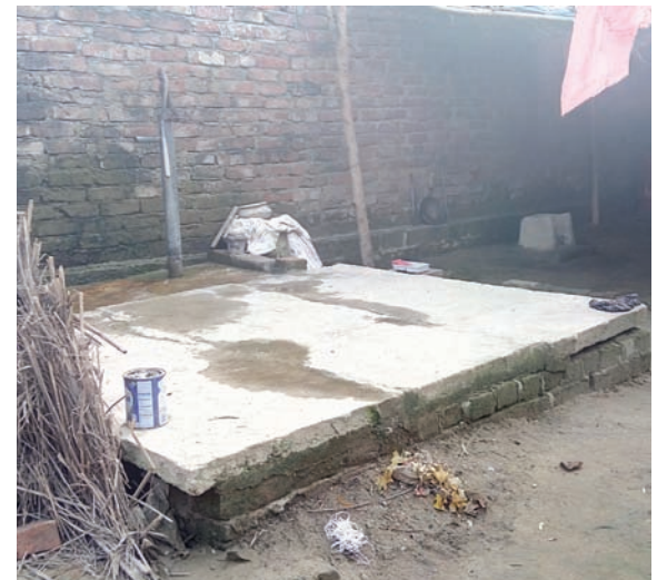
Figure 1: Three chambered septic tank of a household
