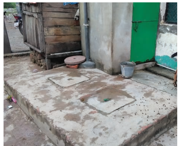
Figure 1: Septic tank having outlet connected to open drain
