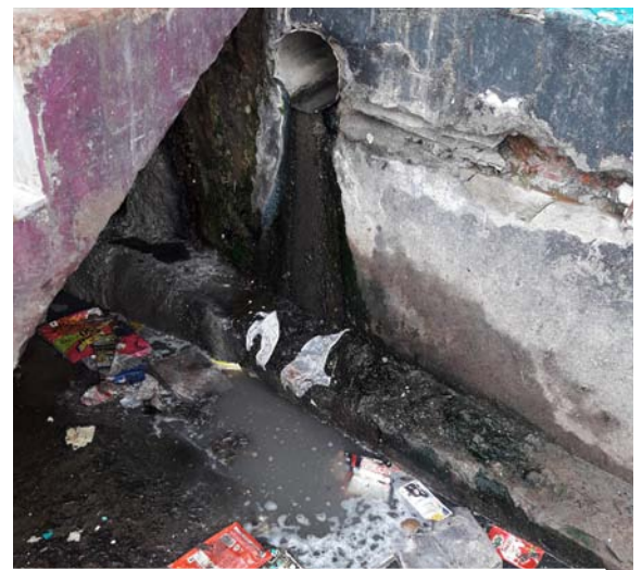
Figure 1: Supernatant of a tank discharges into open drain
