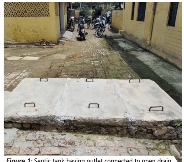
Figure 1: Septic tank having outlet connected to open drain
