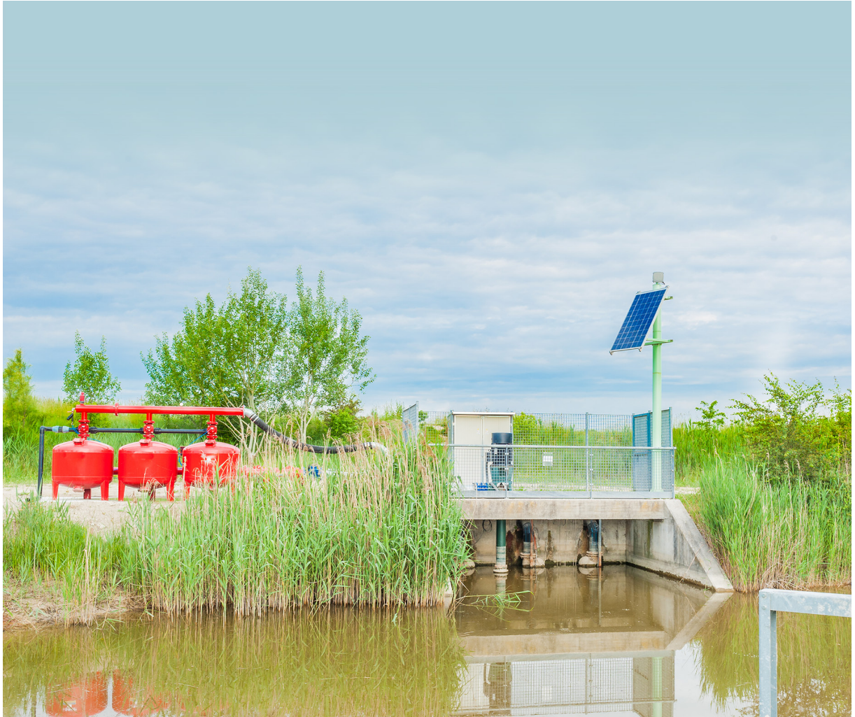
Popularity of solar pumps is increasing with decreasing photovoltaic prices
