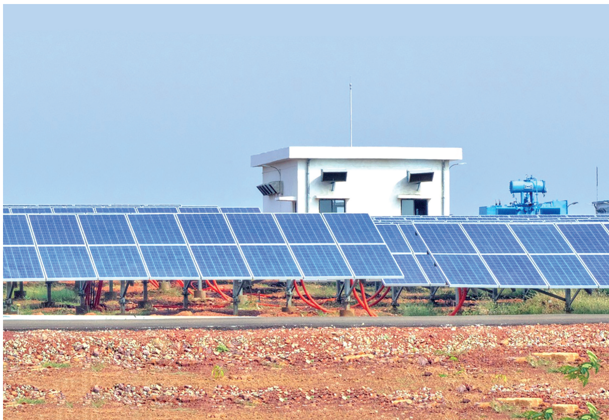
Solarized agricultural feeders turn out to be the most economic of all the alternatives for irrigation
