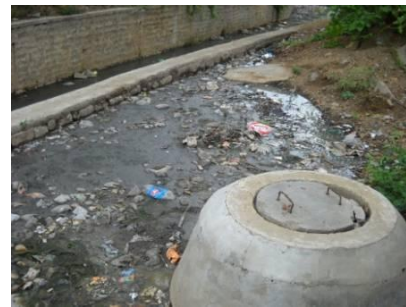
Picture 19: Overflowing manholes
