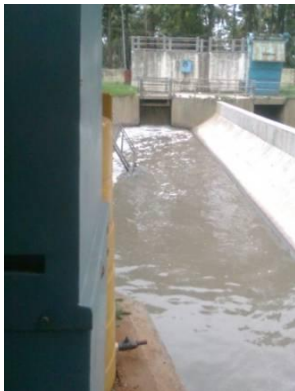
Picture 15: Inlet to STP
