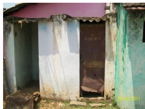
Picture 6: Defunct toilets
