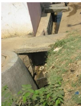
Picture 5: Open drain led to open nala at Gousiyanagar, Ward No. 59
