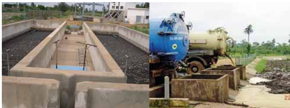
Figure 6.2 Left: the twin settling-thickening tanks of Rufisque faecal sludge management plant, in Dakar, Senegal. The operating cycle lasts two weeks (one week loading, one week desludging), and sludge is transferred to drying beds with a pump. Right: the settling-thickening pond in Achimota, Accra, Ghana, has an operational cycle of 8 weeks (4 weeks loading, 4 weeks desludging). As the sludge is thickened for four times as long, it is not possible to remove it with a pump, and manual extraction is carried out (photo: SANDEC).
