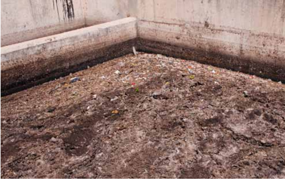
Figure 3.2 Settling tank at Niayes faecal sludge treatment plant in Dakar, Senegal (photo: Linda Strande).
