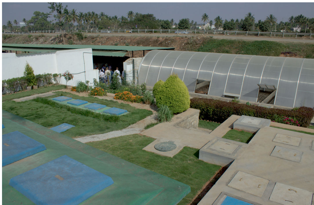
India's first dedicated fecal sludge treatment plant is located in Devanahalli (photo by CDD Society/BORDA).
