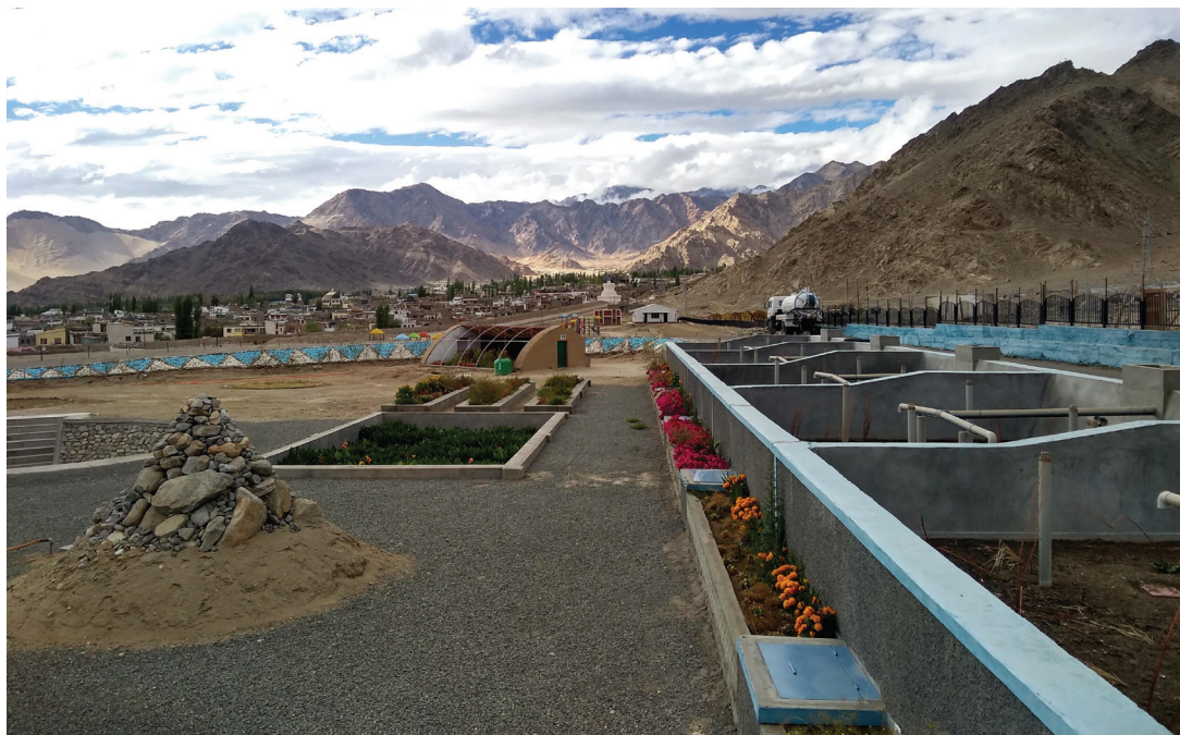
India's first public-private partnership for fecal sludge management services, the fecal sludge treatment plant in Leh (photo by BORDA).
