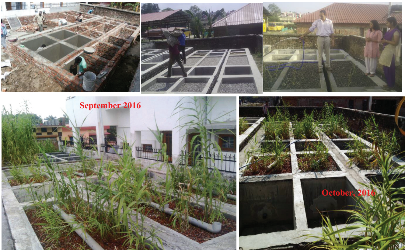
Figure 31: Pictures showing construction of CW units and growth of surface vegetation on CW
