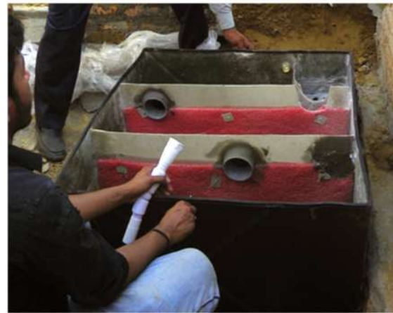
Bio digester section
