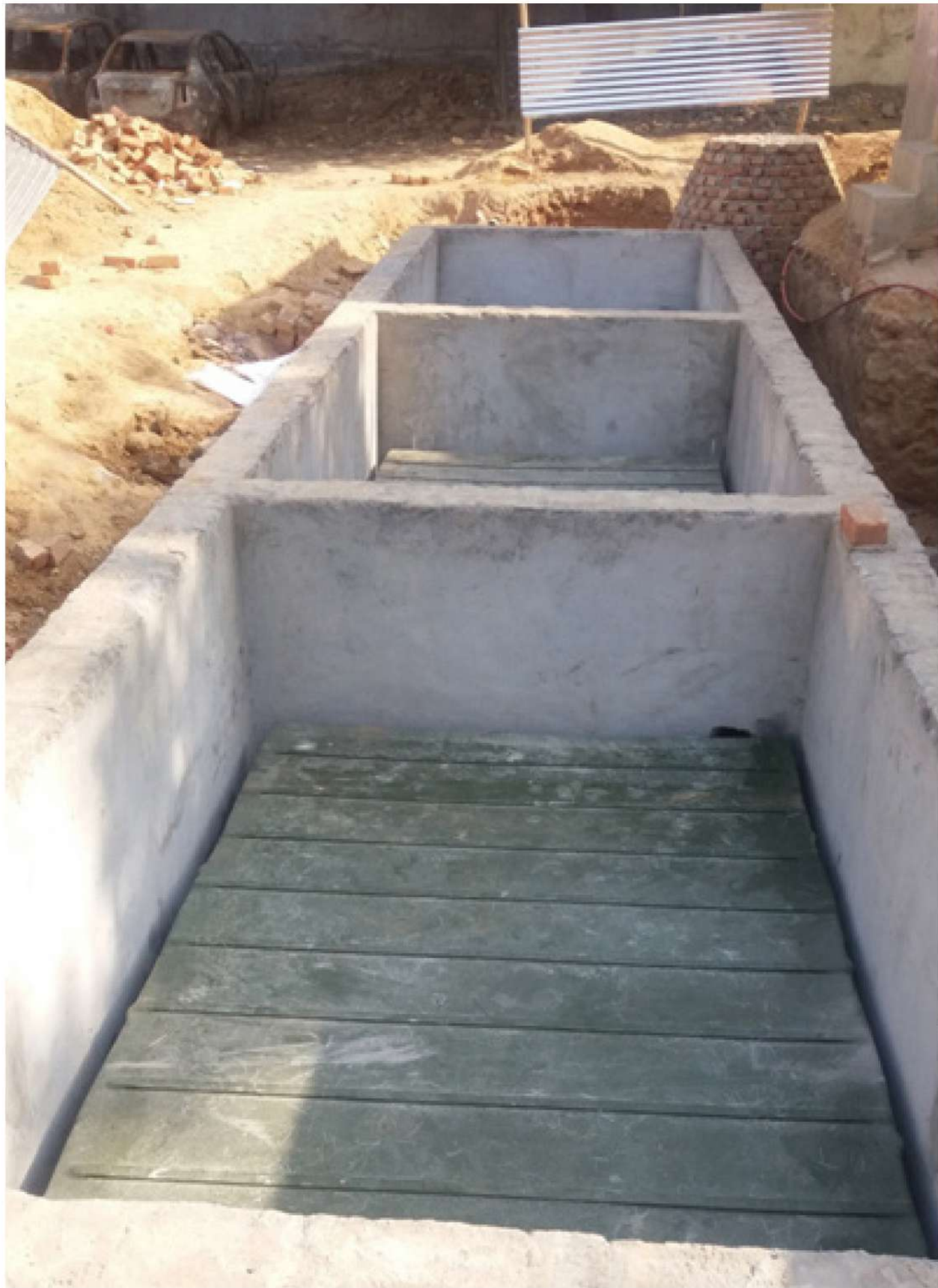
BIO DIGESTER IN PLACE BELOW THE STREET
